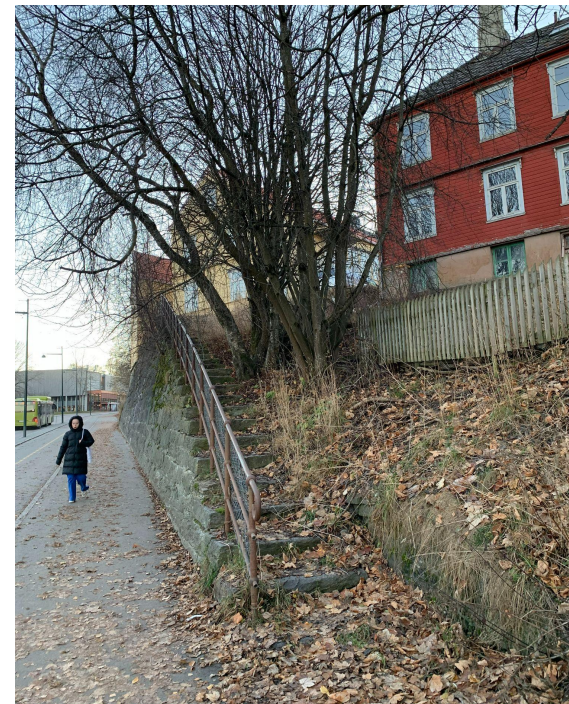
The stairs from Christian Fredriks gate must be upgraded.
